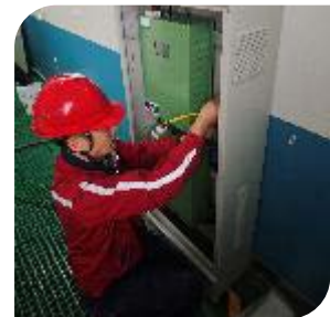
Application of Energy-Efficient Equipment
