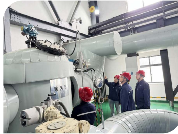
Primary Station Safety Inspection
